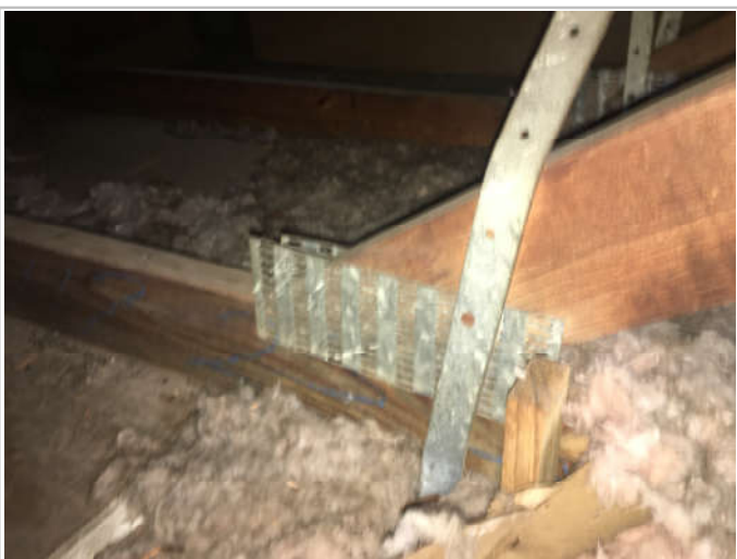
Toe Nail - Not Meeting Nail Requirements
